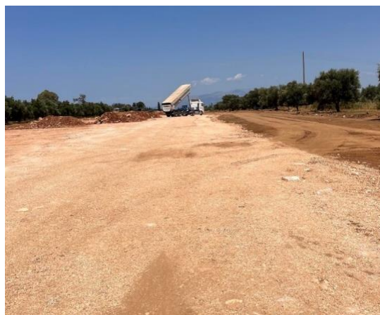
Laying of quarry materials for the replacement of the top soil (k.p.:19+500 – 21+030,00)
