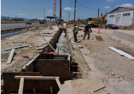
Construction Works for the pipeline Φ800 to the side road of the Motorway
