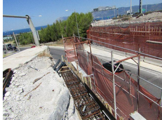
Placement of reinforcement and framework on the abutments, for the placement of the bearings
